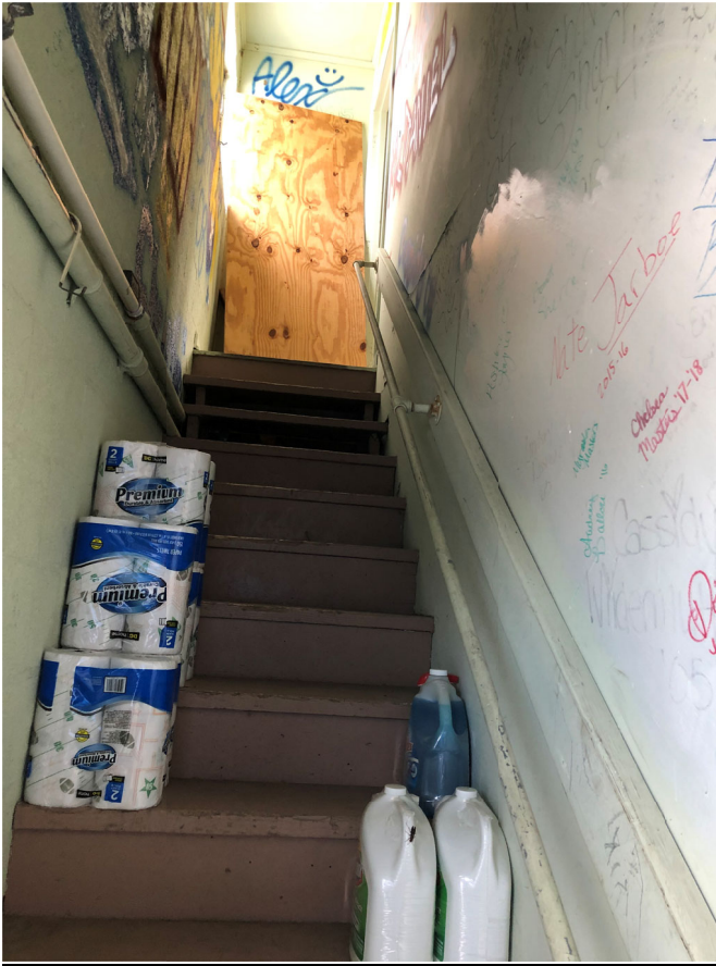
Abandoned upstairs in bathhouse.
