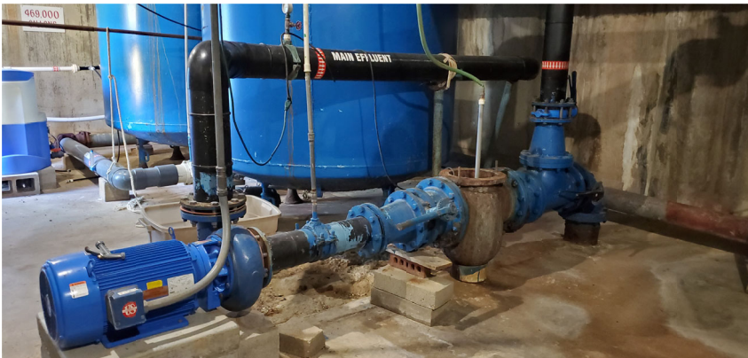
Pump motor, strainer, filter, chlorinator
