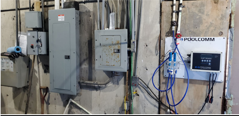
Electrical and Pool Controller.
