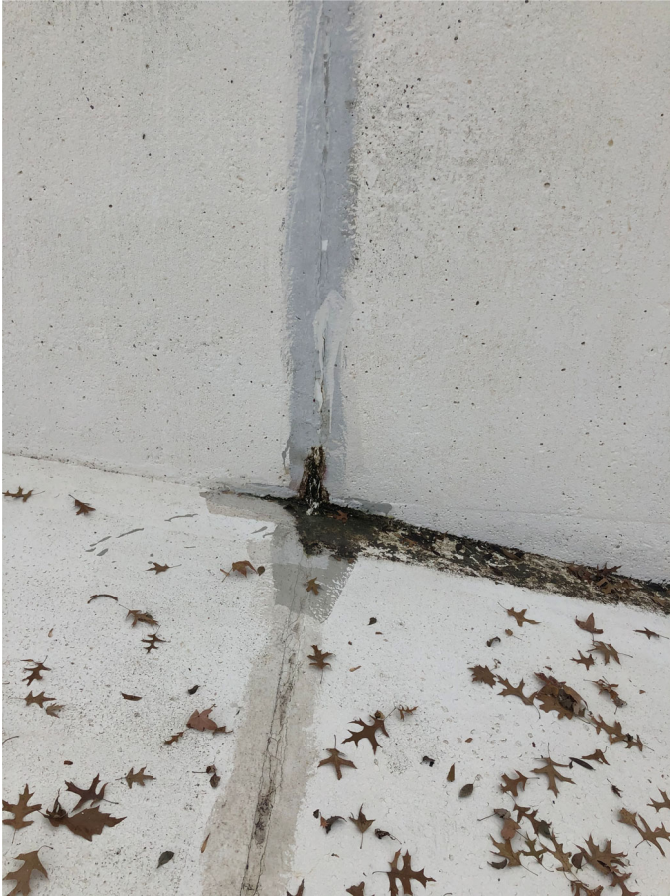
Crack leaching water.
