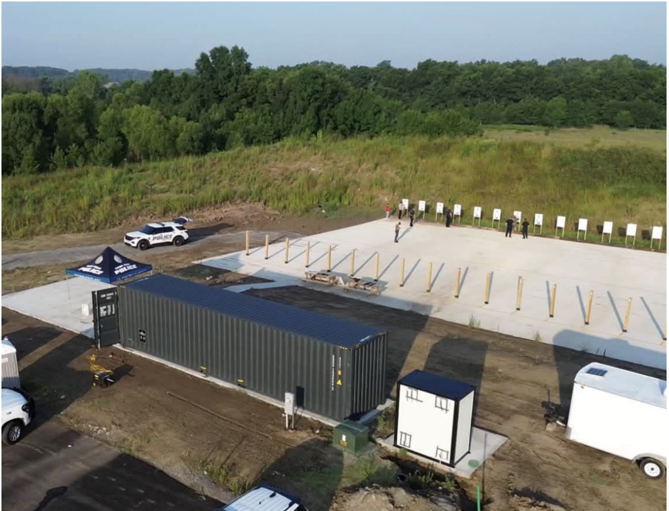
Gray Connex = mini-split installation location
