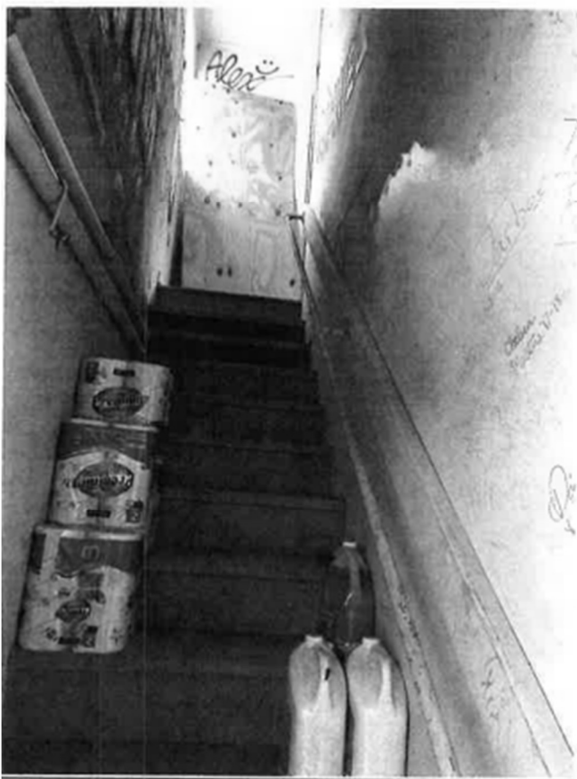
Abandoned upstairs in bathhouse.
