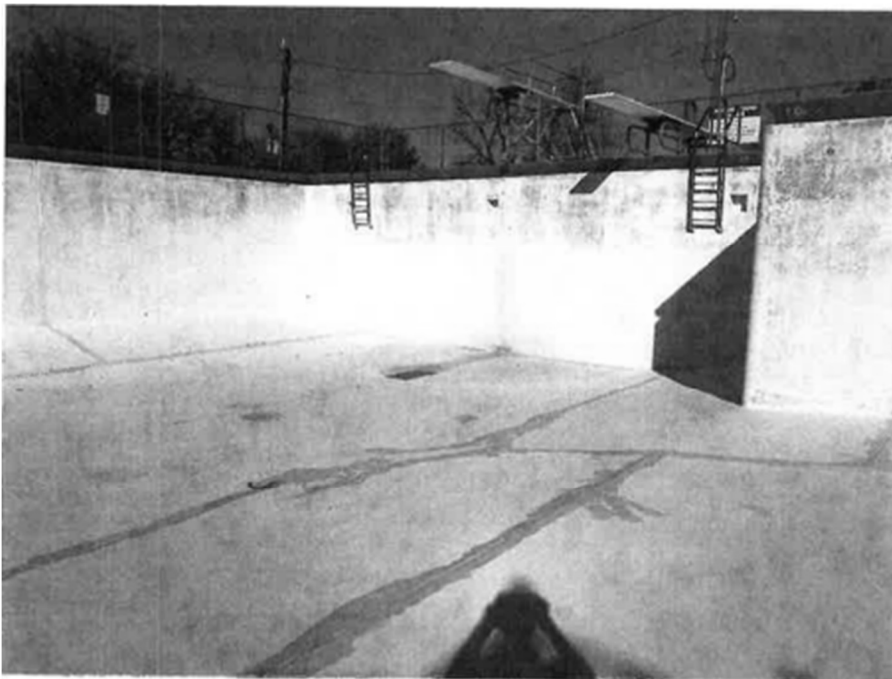
Cracks in deep end floor.
