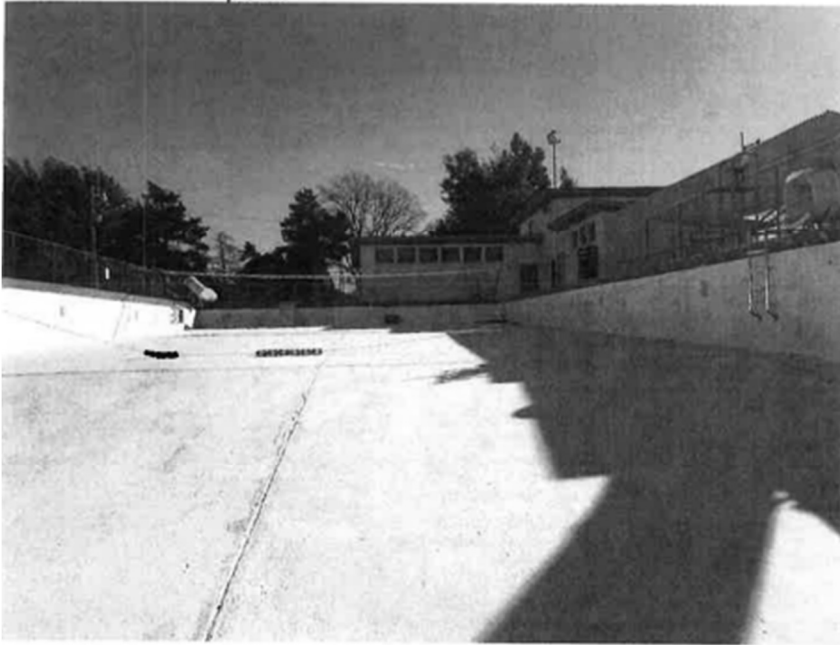
Expansion Joints: The pool is a sectional poured structure. The expansion joints are failing in areas.
